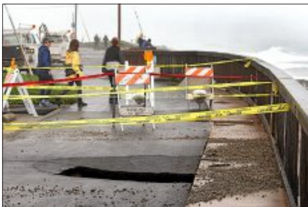
A large sinkhole developed in January on the West Cliff bike path between Woodrow Avenue and Columbia Street due to pounding surf.
