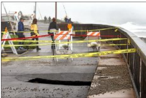
A large sinkhole developed in January on the West Cliff bike path between Woodrow Avenue and Columbia Street due to pounding surf. DAN COYRO — SANTA CRUZ SENTINEL FILE
